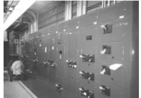
The Pumping Station motor control center with SCADA (Supervisory Control & Data Acquisition System).
