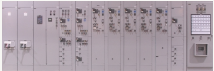
Motor Control Centers
