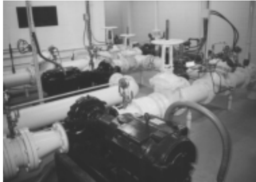
The two new Aurora Booster Pumps and several of the Bermad control valves used in the system.
