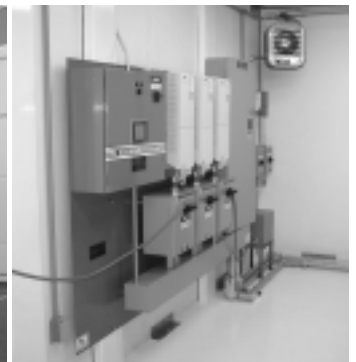
The control panels that operate the system.
