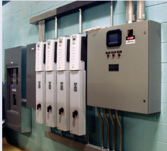
Variable-speed controls operate the lift station with efficiency, saving money on energy costs. Touch screen operation allows push-button control.
