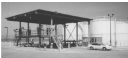
Newly renovated runway deicing fluid facility at Chicago's O'Hare International airport.
