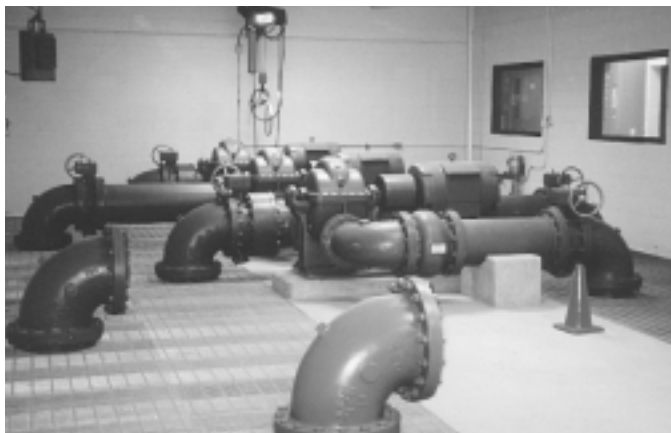
Pump and piping gallery; expandable from three to six pumps.
